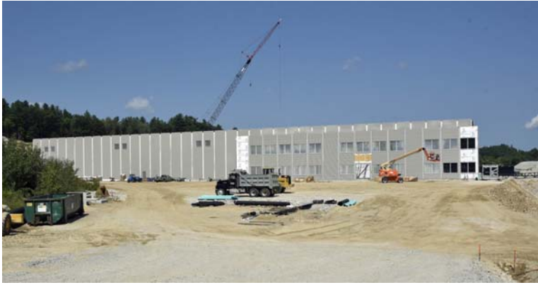
8/26/2018 Coastal Forest Productions Facility under construction - as seen from River Road _DSC1220_edited-1-med7.jpg
