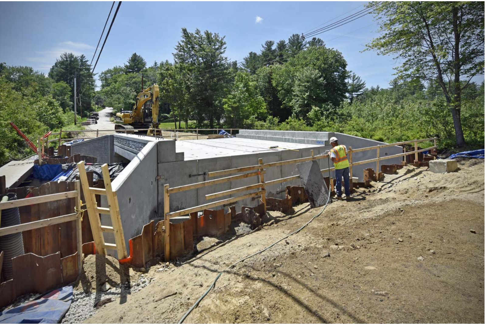
6/12/2018 Bridgedale Bridge at noon after one and one-half days of assembly _DSC1006_edited-1-med7.jpg
