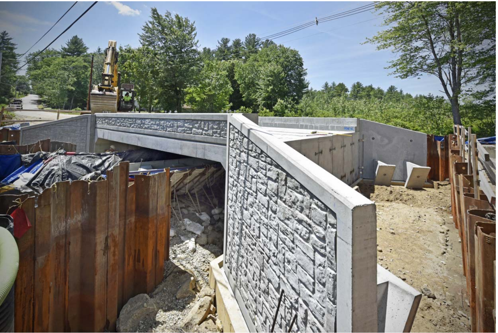
6/12/2018 Bridgedale Bridge at noon after one and one-half days of assembly _DSC0998_edited-1-med7.jpg
