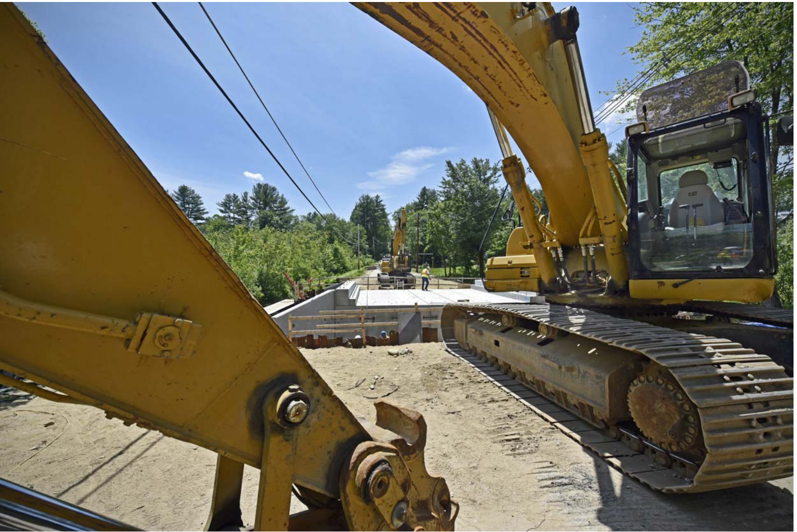
6/12/2018 Bridgedale Bridge at noon after one and one-half days of assembly _DSC0992_edited-1-med7.jpg
