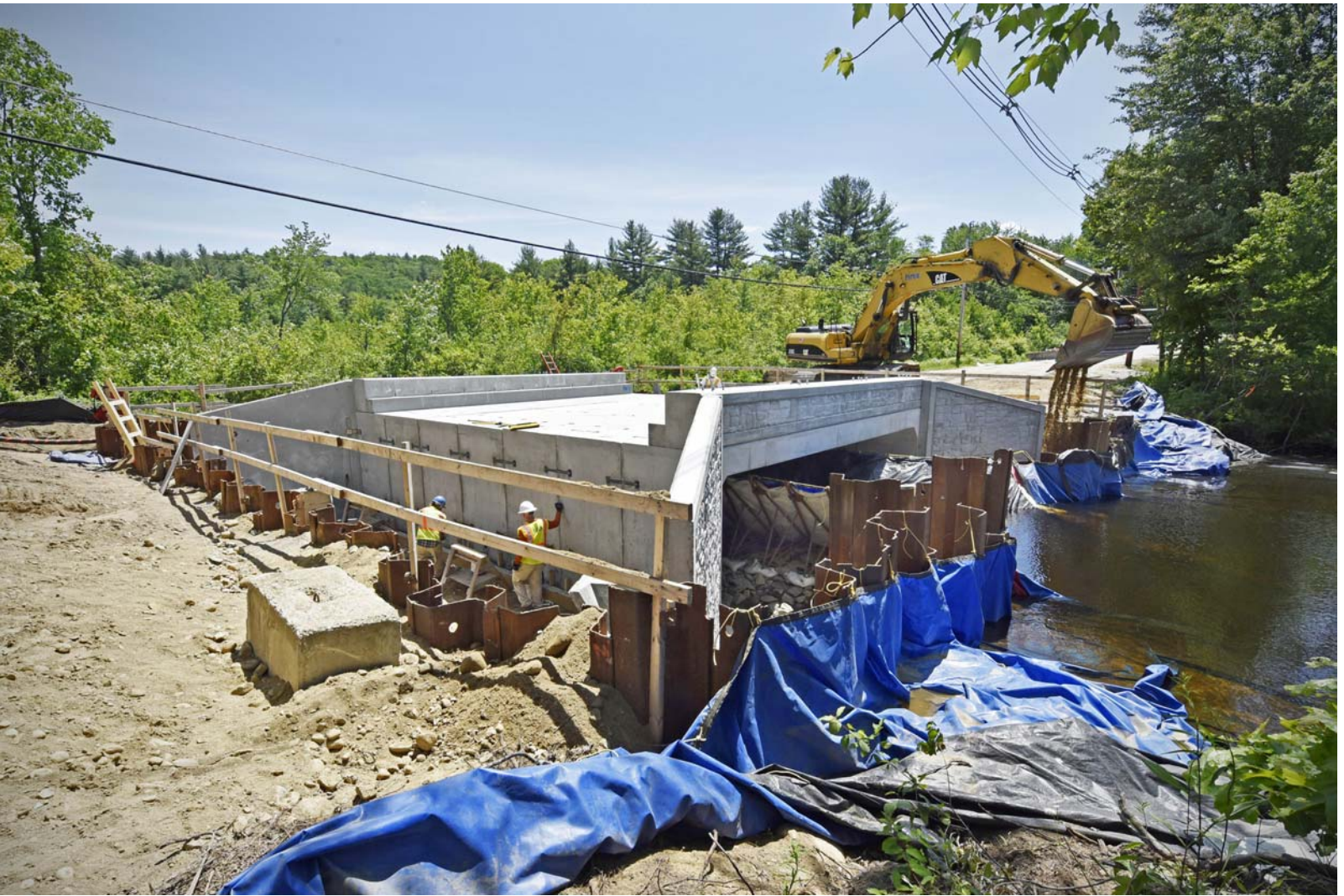
6/12/2018 Bridgedale Bridge at noon after one and one-half days of assembly _DSC0986_edited-1-med7.jpg
